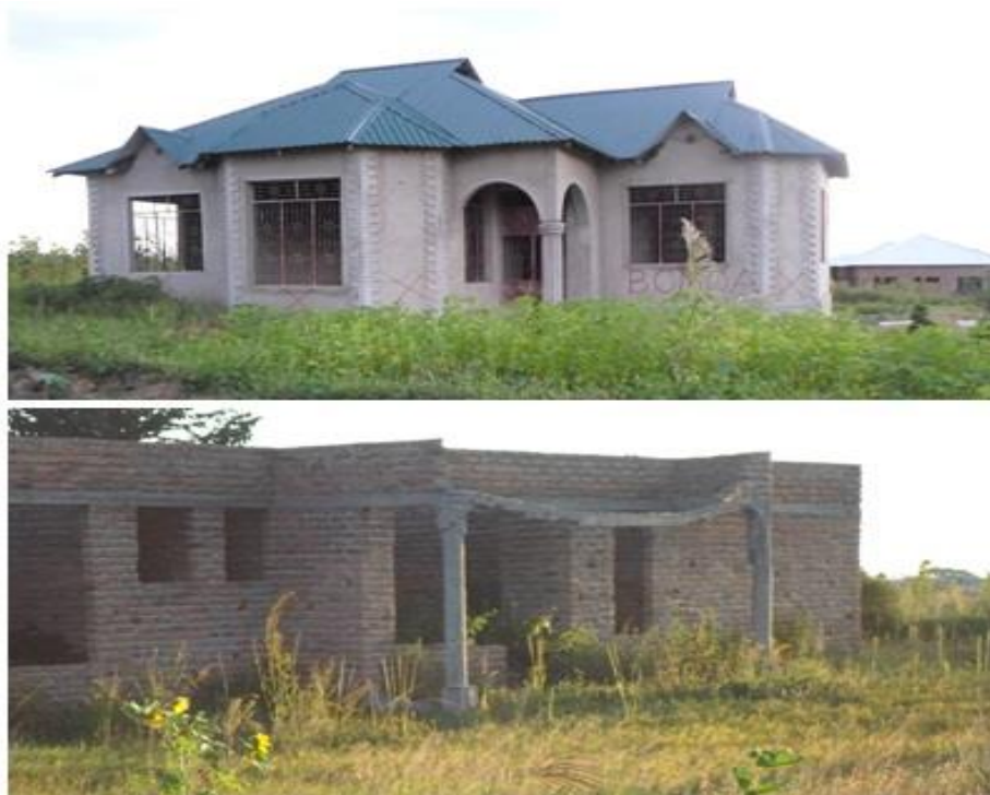
Plate 5.1 Lack of regular supervision and inspection
